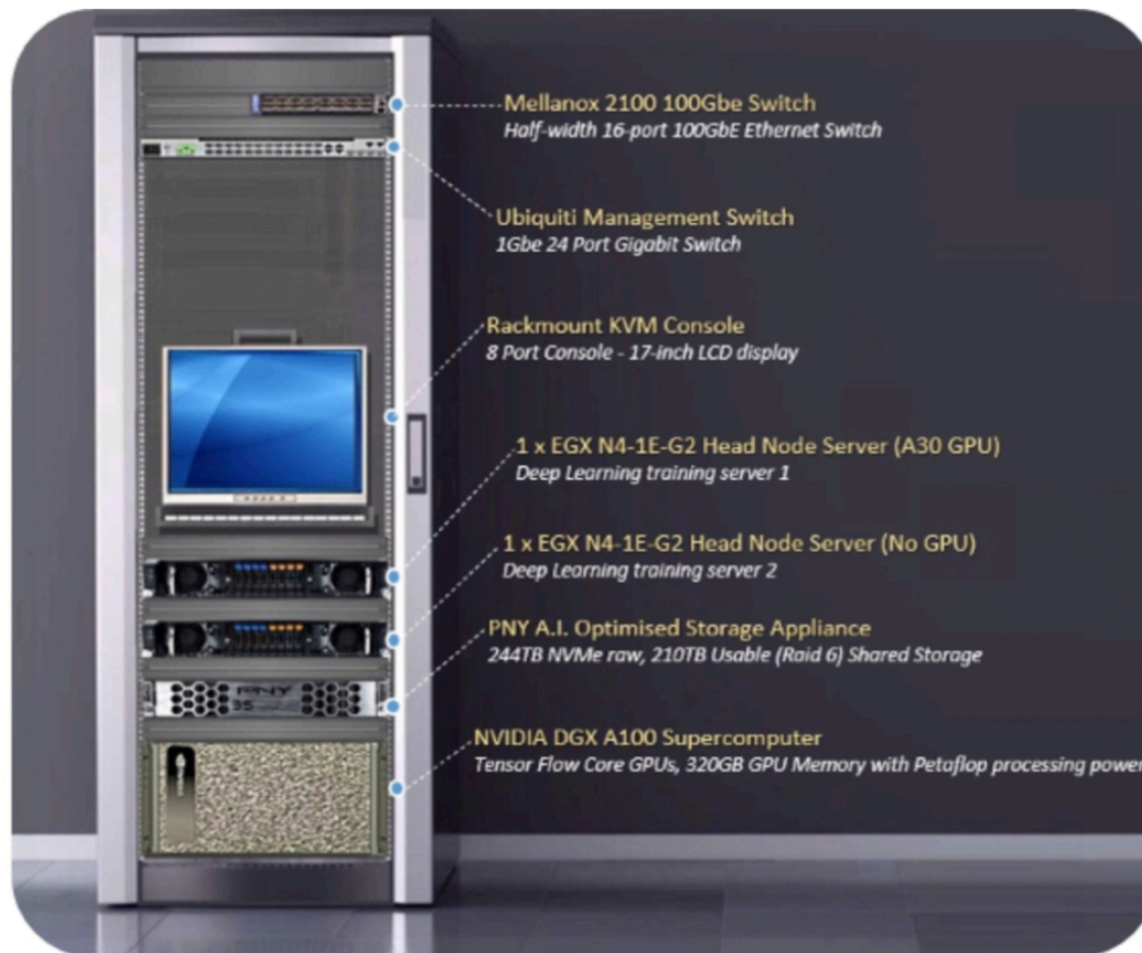
Figure 2: AIC on site infrastructure, currently installed in 7 NHS Trusts
